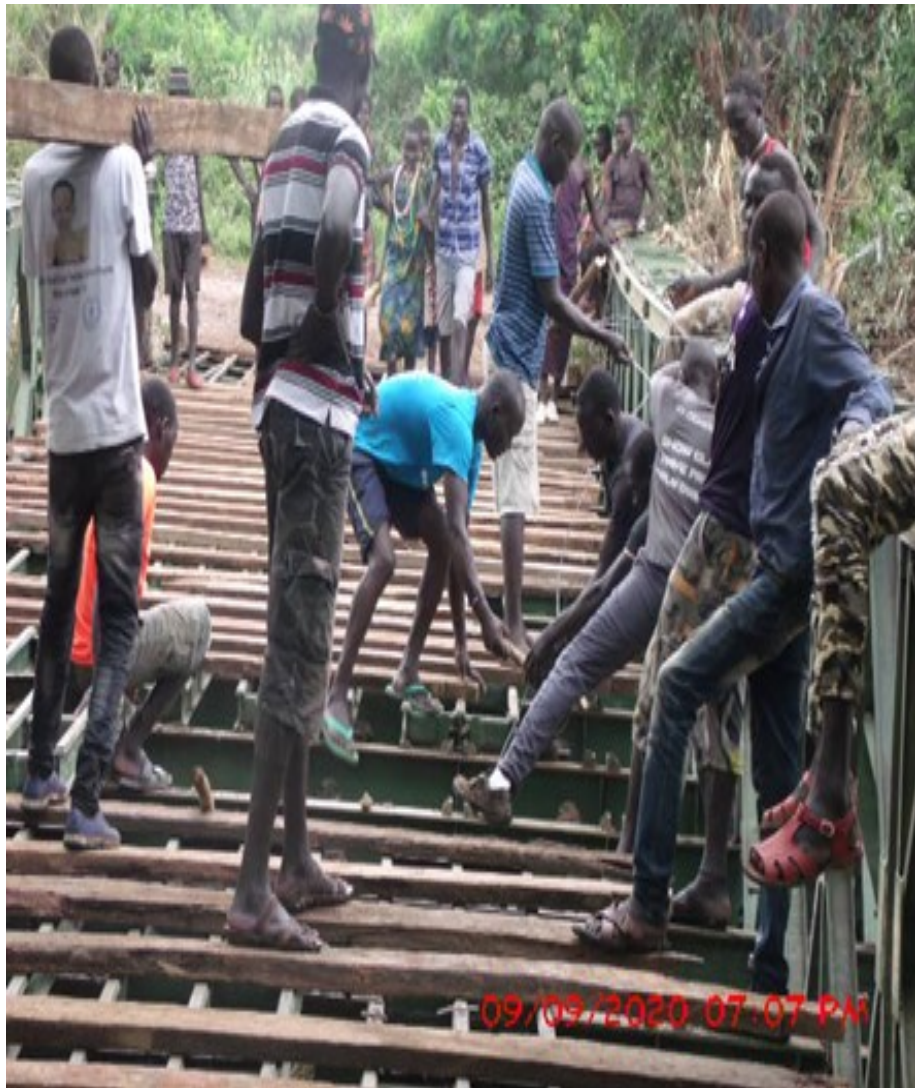
The staff and community in Kuron struggles to fix some of the broken parts of the bridge destroyed by floods in September 2020
