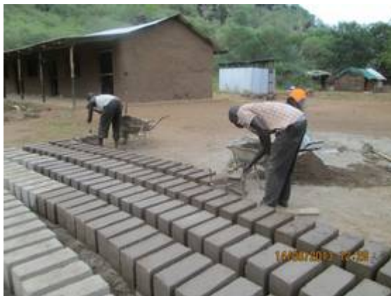
Contractor John Ochan producing quality blocks for teachers' houses. A total of 1200 blocks have been produced. 3,800 more needed.
